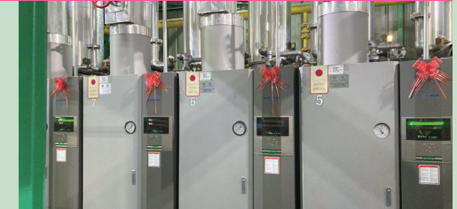
Once-through Boiler (Indonesia) DIC Corporation
